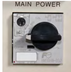
FIGURE 3-15 Compressor main power switch in off position
